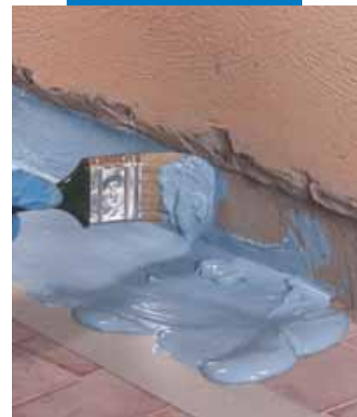
Application of Mapelastic® AquaDefense by brush between floor and wall before applying Mapeband
